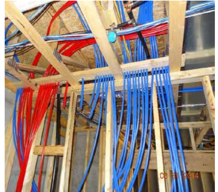
Example of a very large home-run plumbing system
